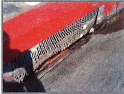
Figure 3.8 Typical opening cover after Rain Event No. 4 (3/19-20/06)
