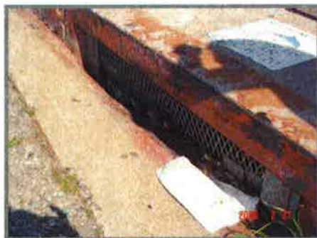
Figure 3.7 Typical opening cover after Rain Event No. 3 (2/17-18/06)
