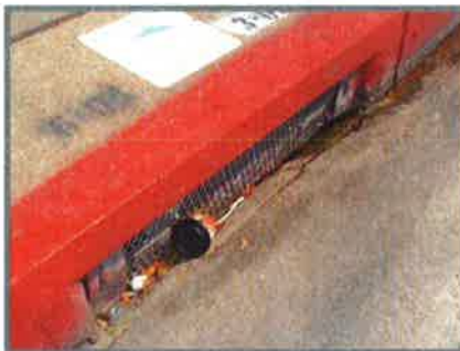
Figure 3.10 Typical opening cover after rain event less than 0.25in (4/4-5/06)
