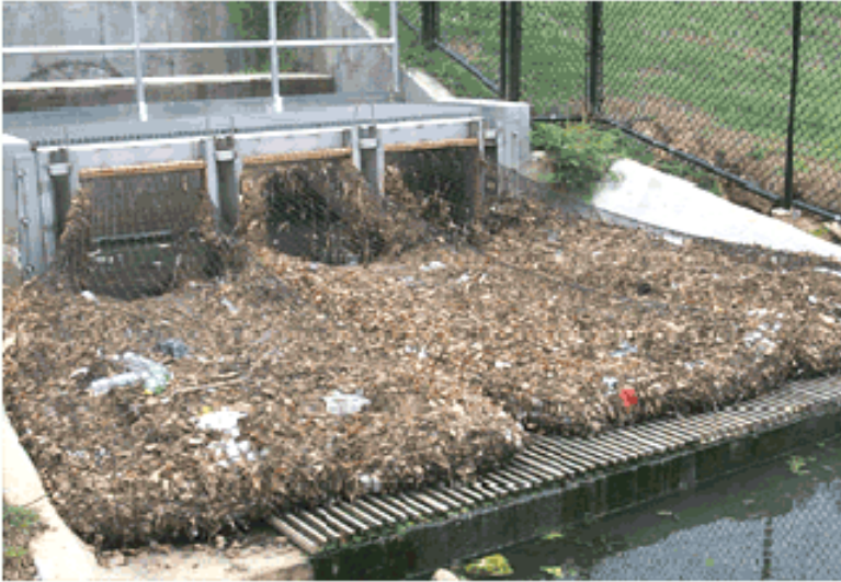
End of Pipe unit collects trash in nets after storm in a city park.
