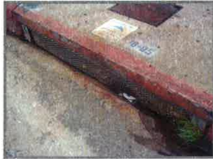
Figure 3.5 Typical opening cover after Rain Event No. 1 (10/17-18/05)
