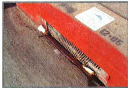
Figure 3.6 Typical opening cover after Rain Event No. 2 (12/31/05 – 01/02/06)
